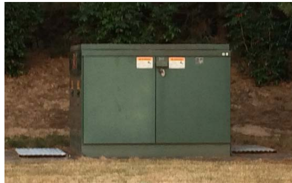
Typical of sectionalizing switch
