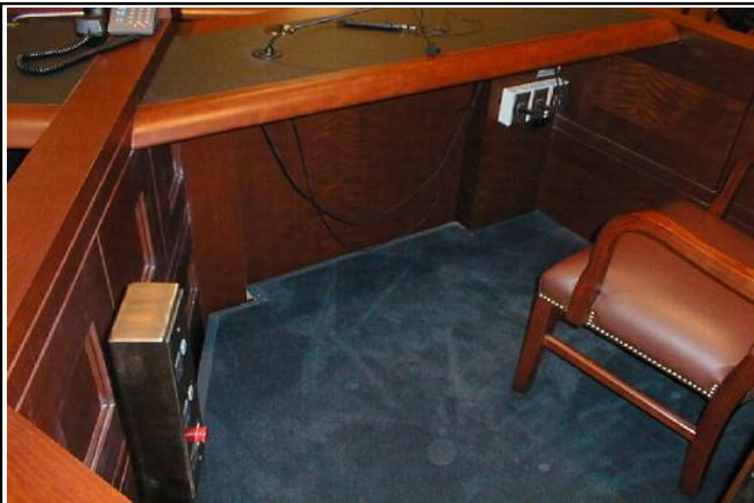
Irregular Edge Of Platform Results In Large Gaps
