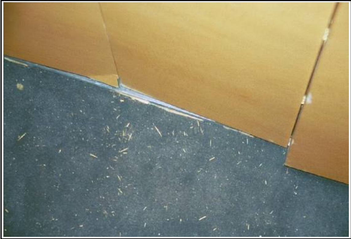
Damaged Folding Panels
