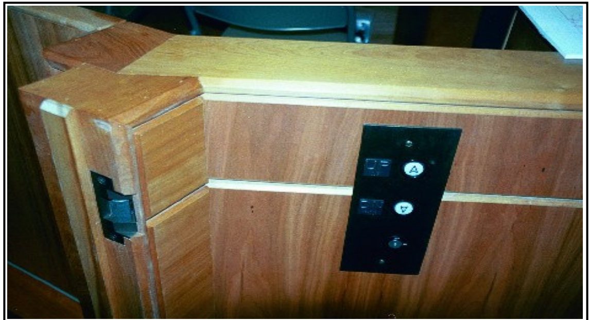
Controls At Courtroom Well Level
