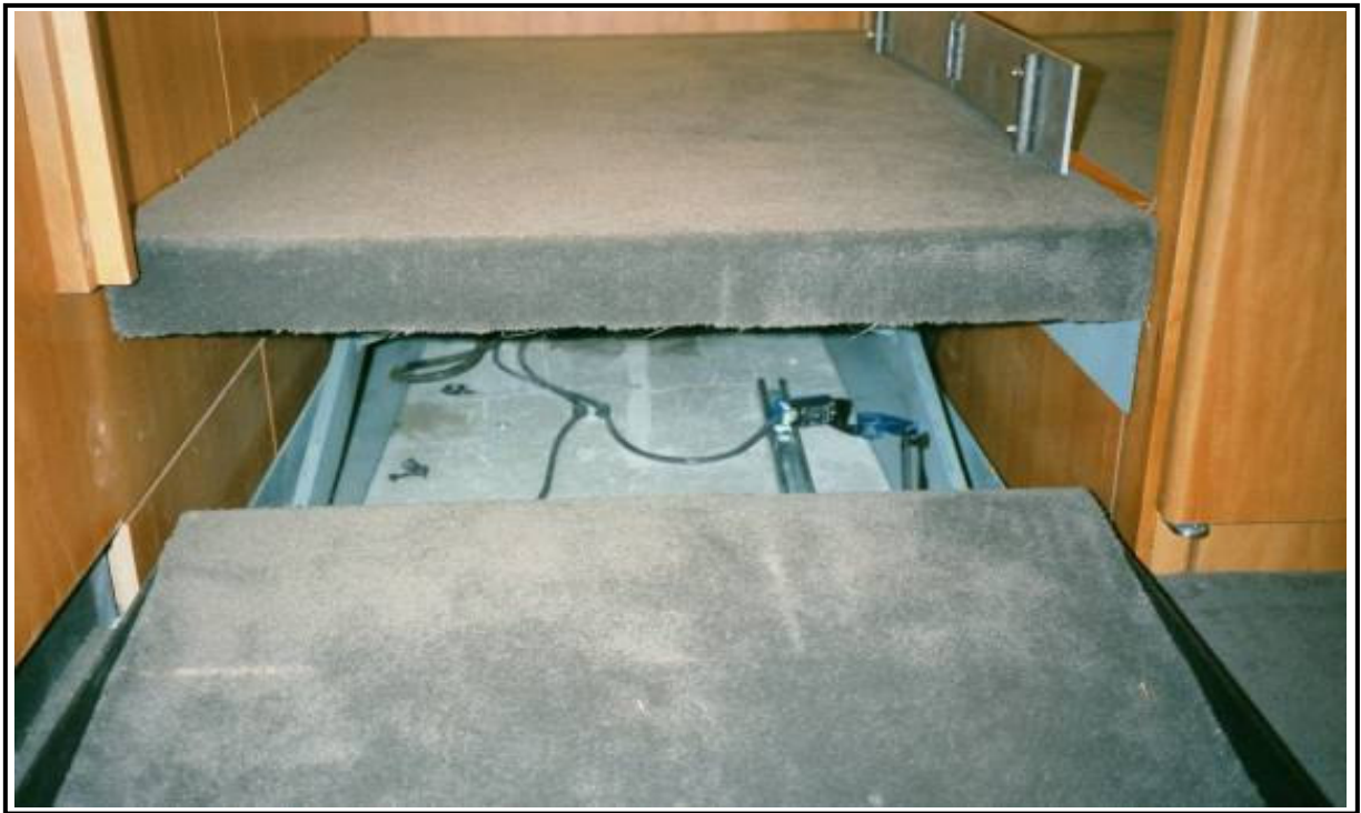
Lift With Manually Installed Wheel Stop And Ramp In Foreground
