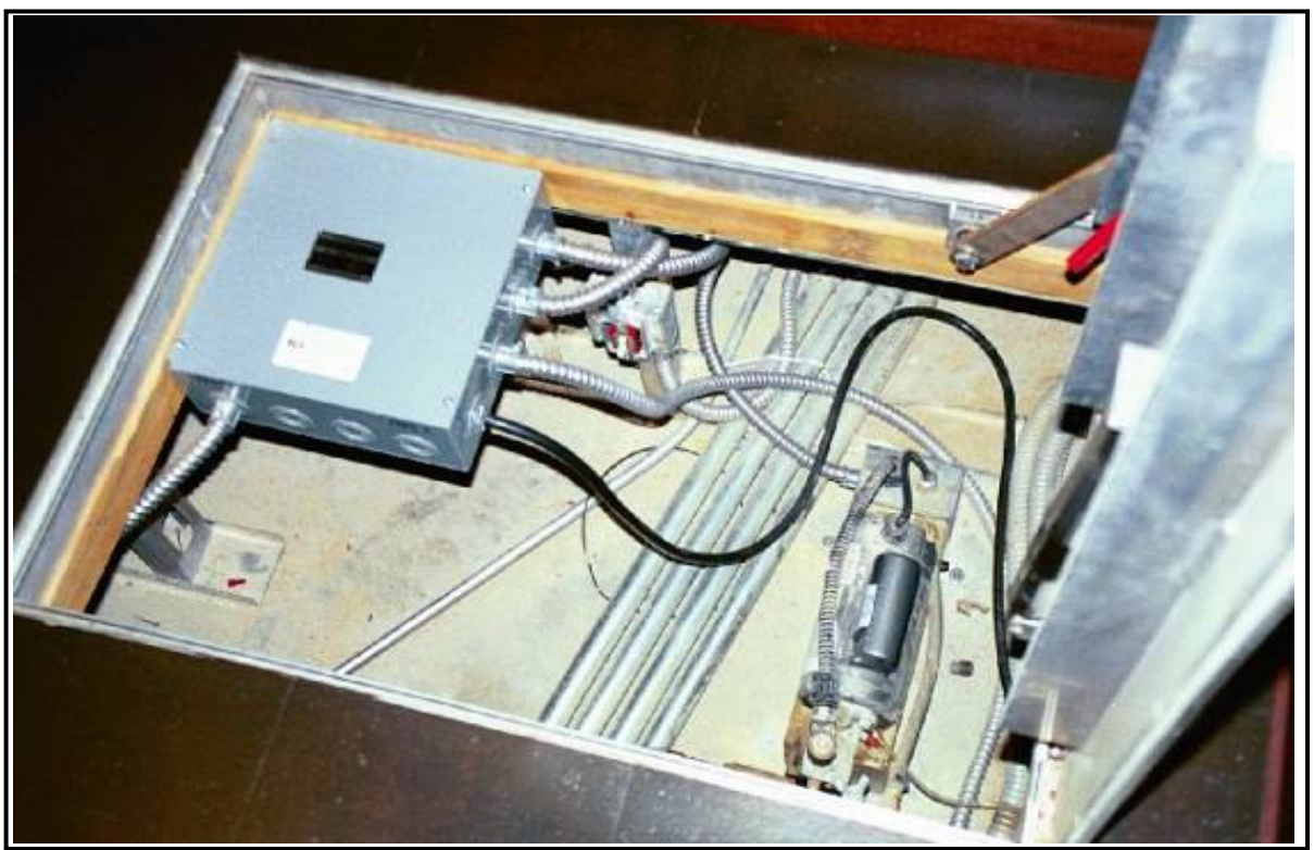
Access Area With Electrical Panel And Hydraulic Pump
