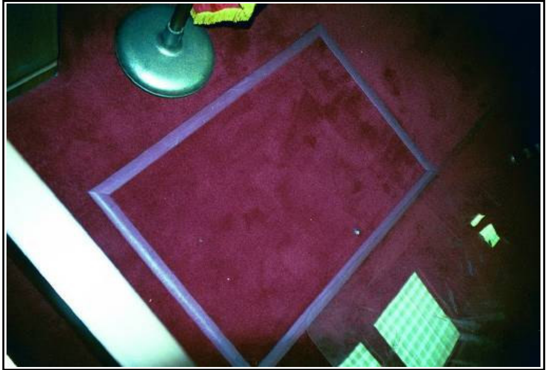
Access Panel To Lift Motor And Electrical Control Panel At Judge's Bench Floor
