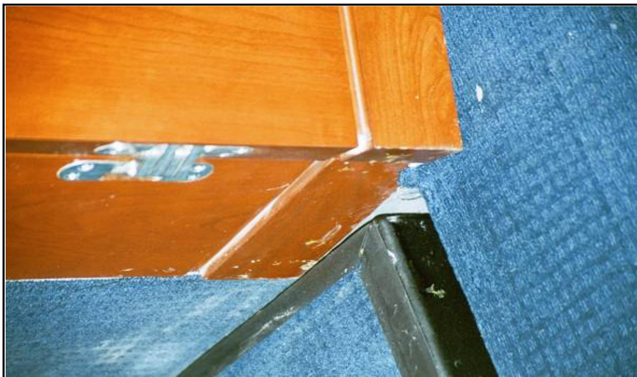
Gaps At Lift Edges
