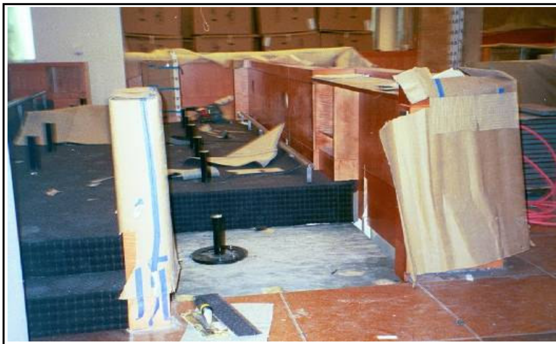
Jury Box Unit At Courtroom Well Level
