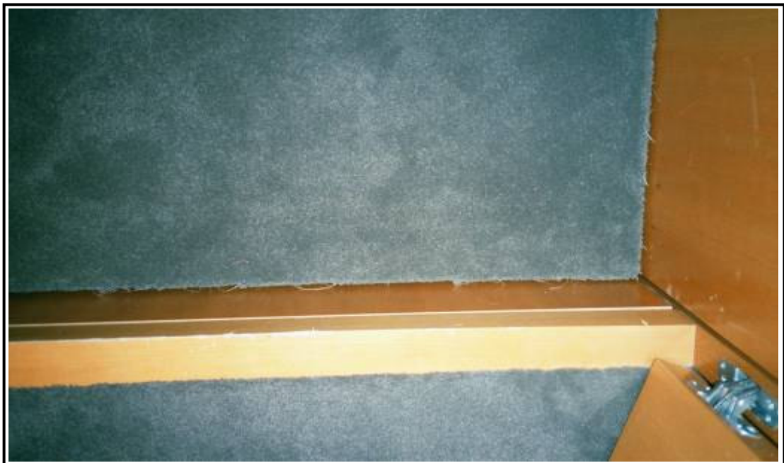
Platform Carpet Cover With Frayed Edges
