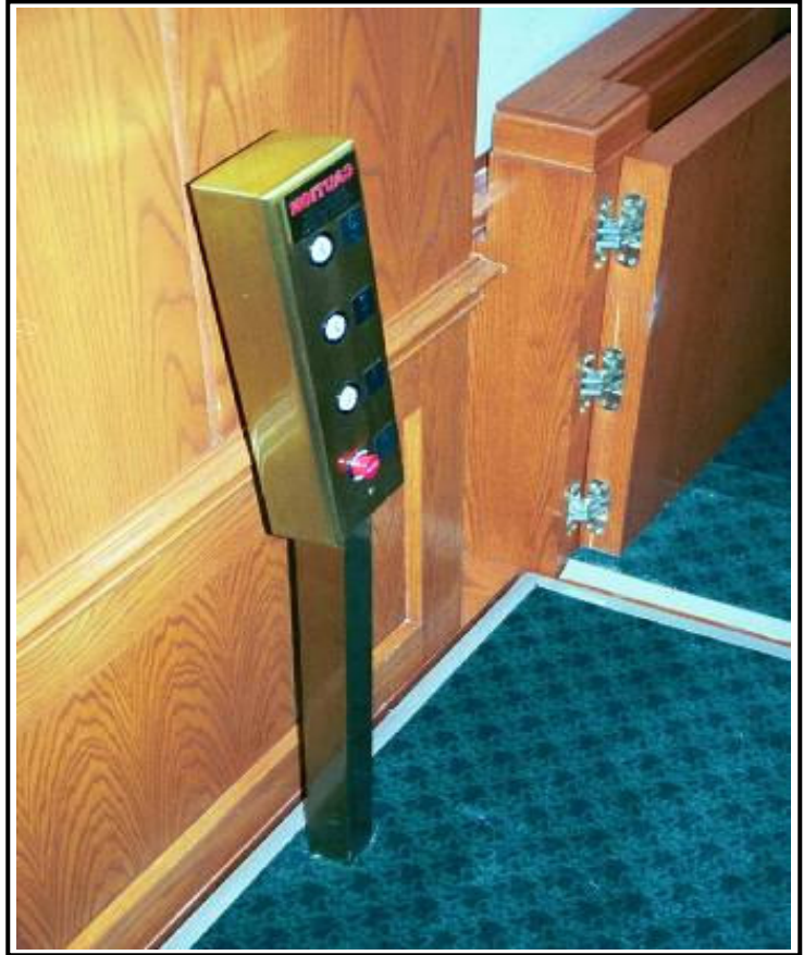
Lift Controls On Platform
