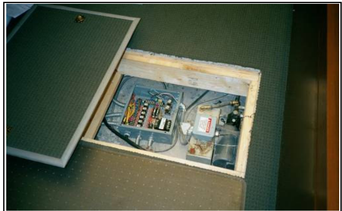
Access To Electrical Panel At Hydraulic Pump In Judge's Bench Floor
