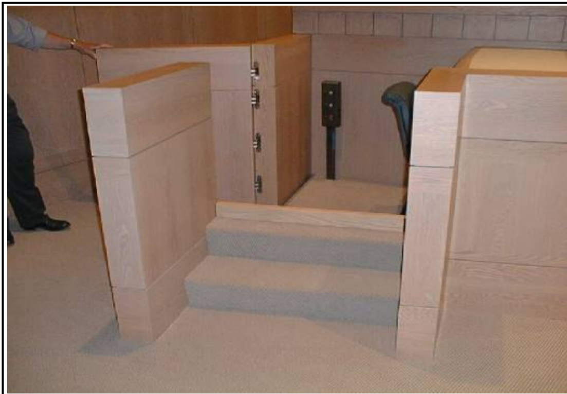
Note: Board Placed Manually As Barrier At Steps
