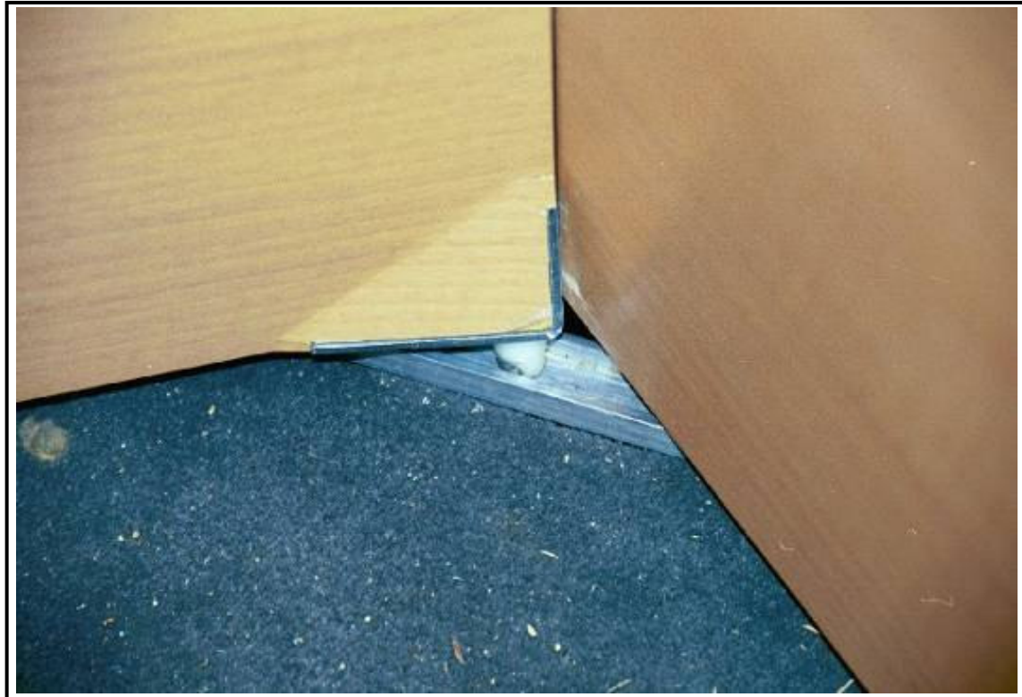
Close-up Of Damage
