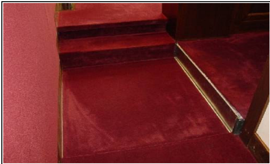
Lift At Lowest Level
