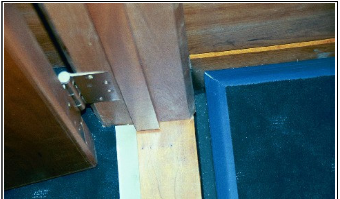
Large Gap Between Lift At Enclosure
