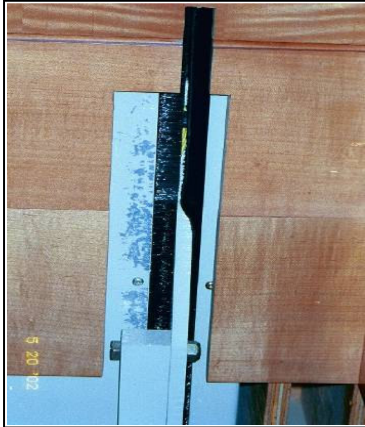
Carriage Frame Protruding Through Enclosure
