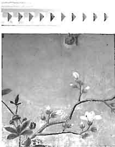
Figures 14 and 15 (above left and immediately above). In the Dillon Room at Blair House, Washington, DC, side-mounted sprinklers have escutcheons painted to match existing historic wallpaper.
