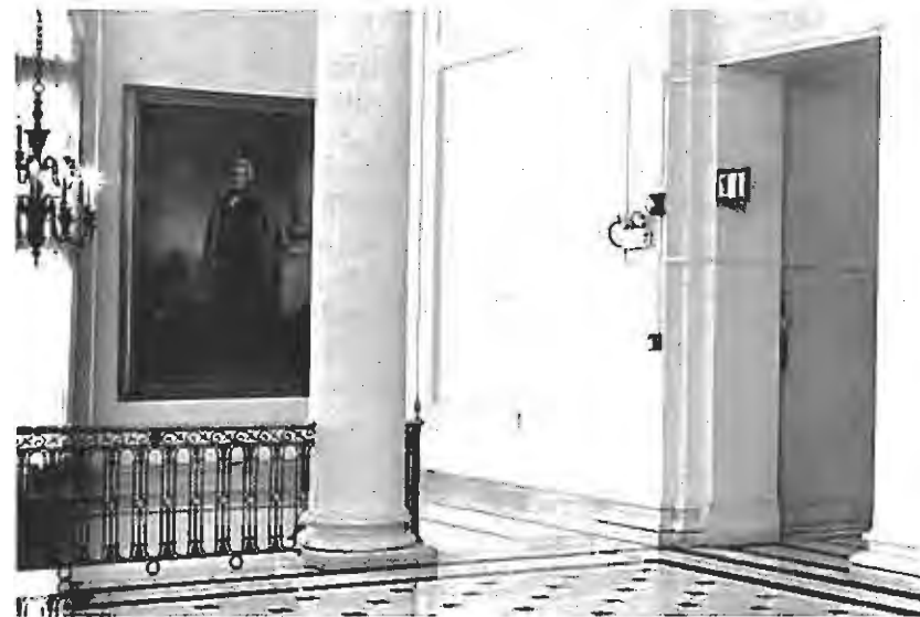
Figure 18 (above right). This sprinkler piping, fire alarm wiring and emergency lighting could have been installed in the wall to create less of an impact on the historic fabric.
