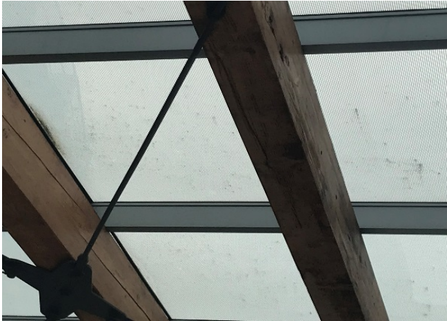
The low slope on this canopy does not permit rain to clean the glass adequately. Below, a new laminated glass unit has cracked.
