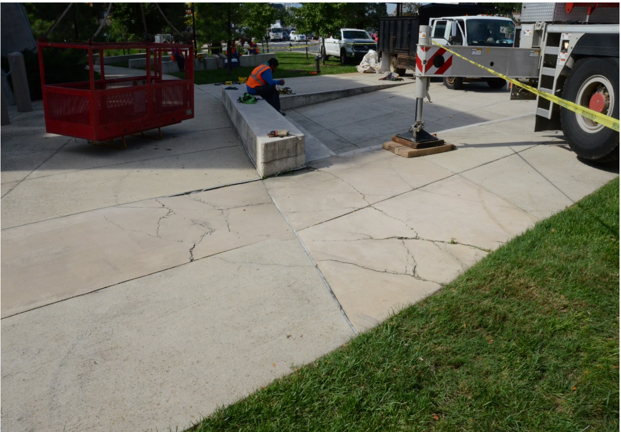
Specify plazas for durability, with stone selections that have good track records for a given geographic area.
