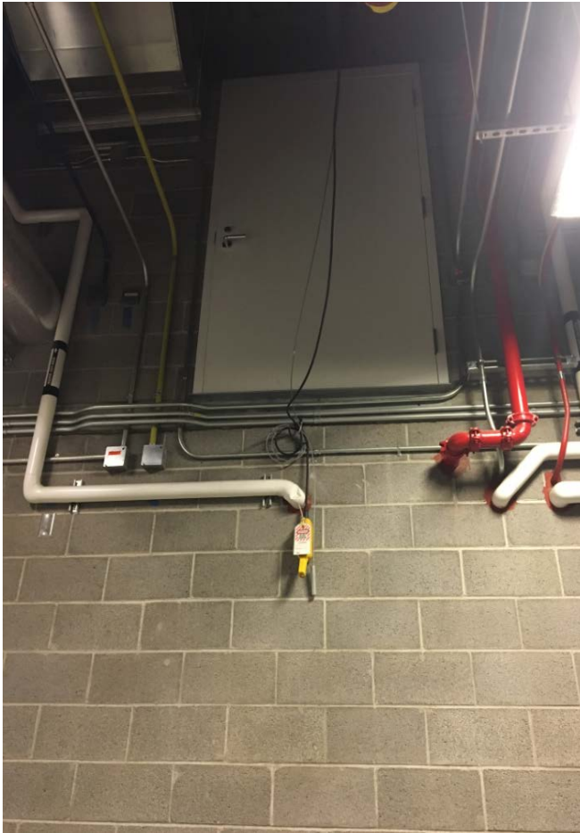
Avoid single leaf doors for areas that need equipment delivery and removal.
