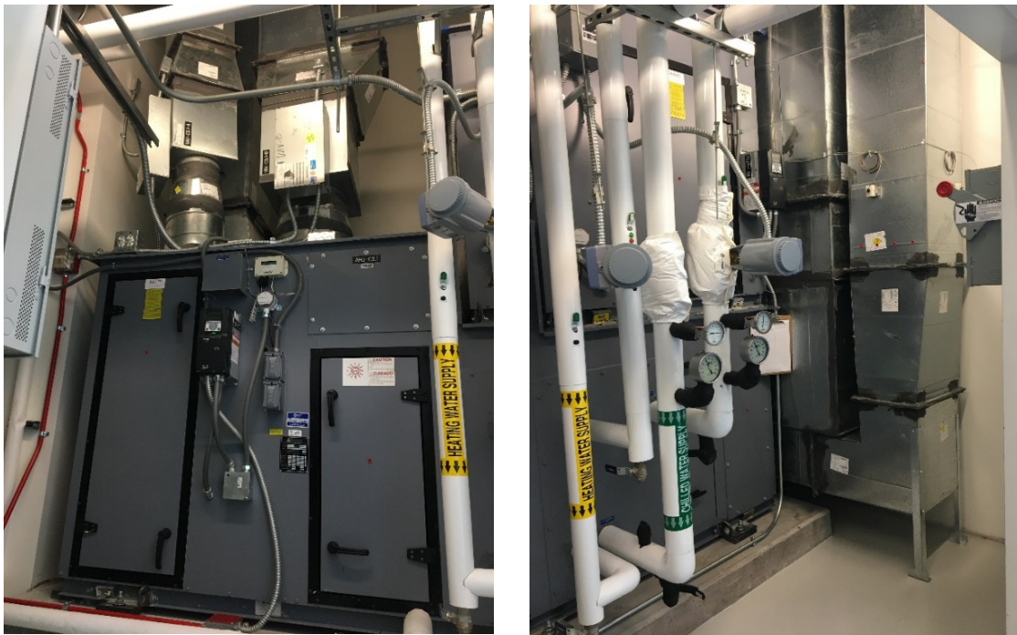
VAV boxes directly above the Air Handling Units allow for easy access for maintenance.
