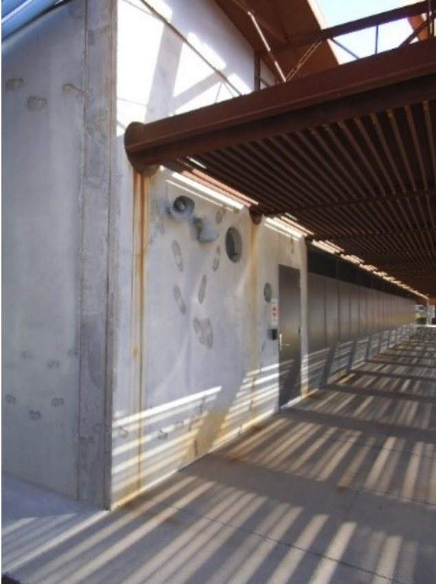
Rundown staining caused by rusting steel.
